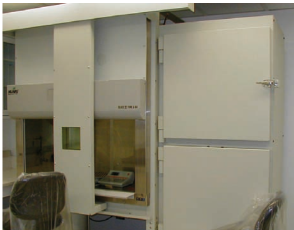
FIG. 4.3. Two mini-cells next to a laminar flow cell in a new PET installation.
