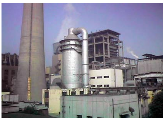
FIG. 2. Flue gas cleaning plant in Chengdu, China.
