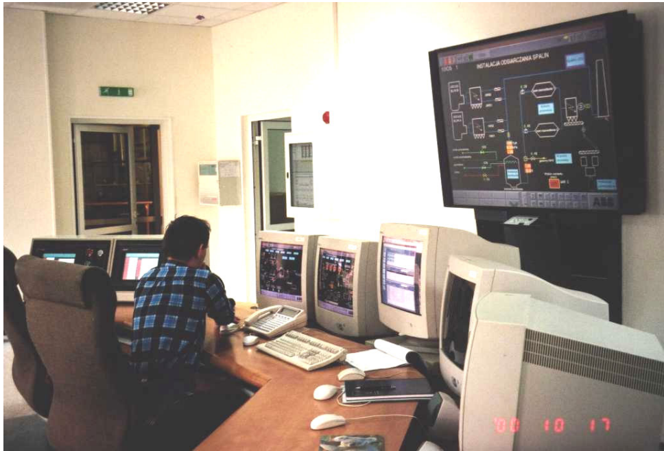
FIG. 5. Control room at EPS Pomorzany.
