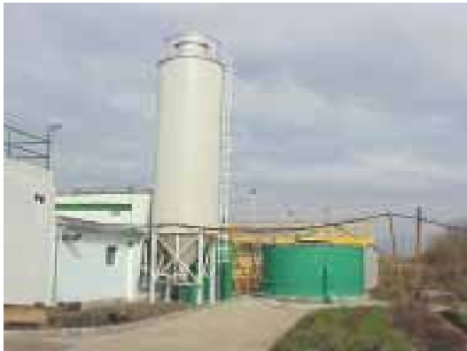
Chemical reactor with lime container
