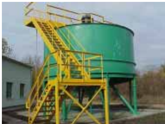
Collecting tank for the underflow
