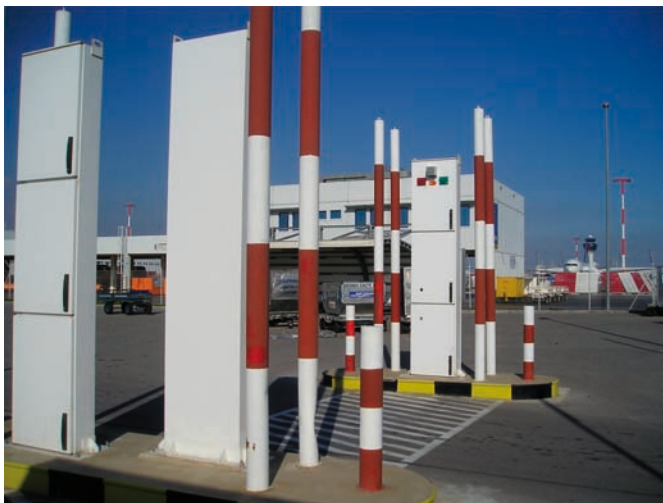
FIG. 16. Vehicle monitors installed at a border crossing.
