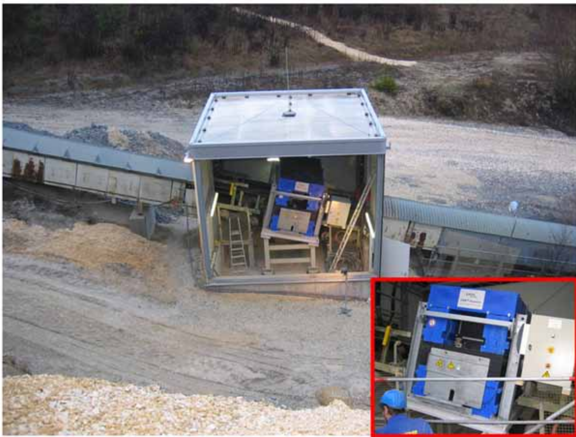
FIG. 9. SODERN Neutron analyser on a cement plant conveyor belt – Allmedingen, Germany (Schwenk Courtesy).
