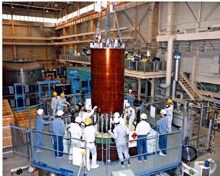
FIG. 6 Installation of the CS Insert Coil into the inner bore of the CS Model Coil
