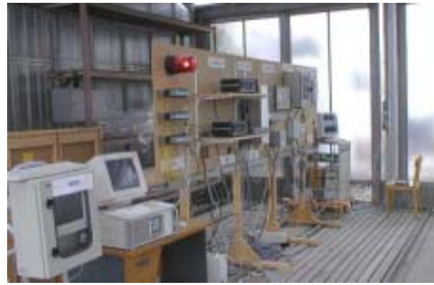
FIG. 3. View of the control units of the detector systems and the ITRAP lab test control system
