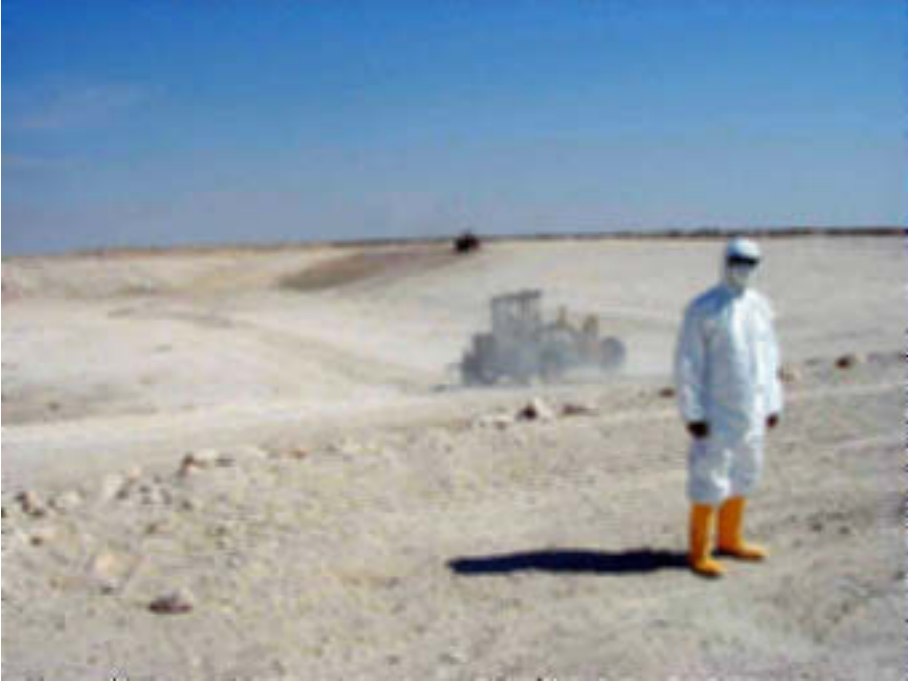
FIG. 29. Remediation of contaminated land after drying the lagoon (courtesy: Atomic Energy Commission of Syria).
