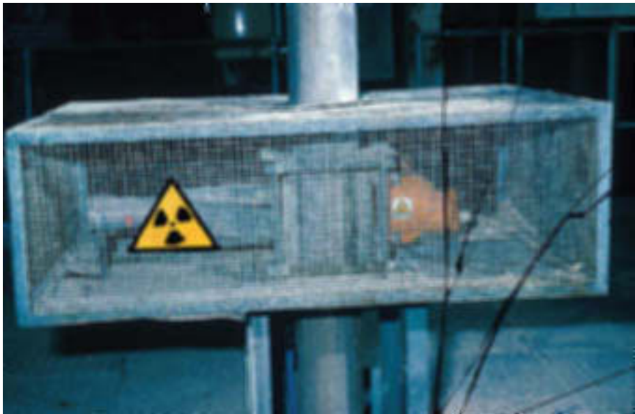
FIG. 5. Installed density gauge (courtesy: National Radiological Protection Board, UK).
