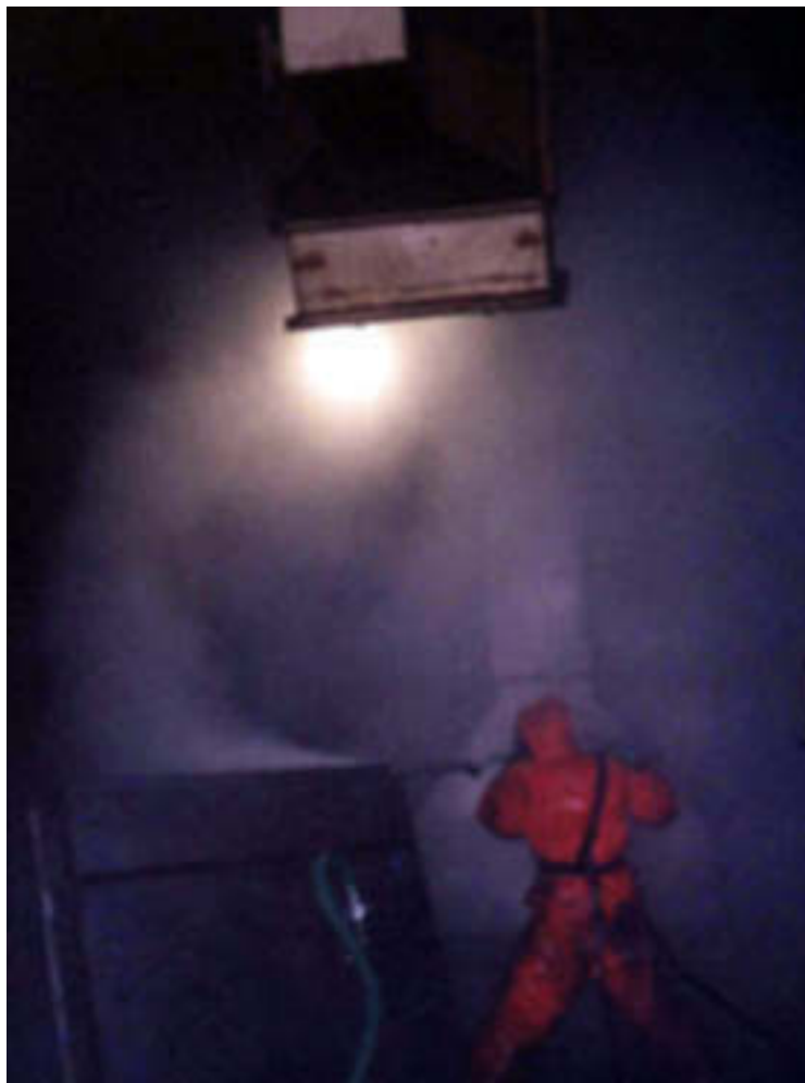
FIG. 36. Workers using HPWJ lance (overhead extractor removes airborne contamination) (courtesy: Atomic Energy Commission of Syria).
