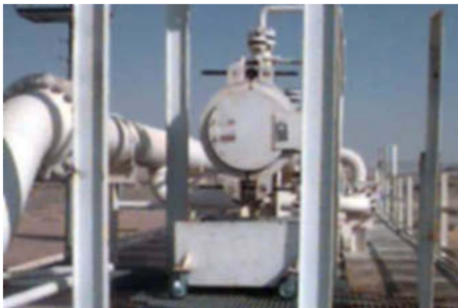
FIG. 4. Pipeline pig trap (courtesy: Atomic Energy Commission of Syria).
