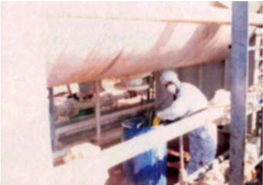
FIG. 34. Removal of bulk sludge from a vessel (courtesy: Atomic Energy Commission of Syria).
