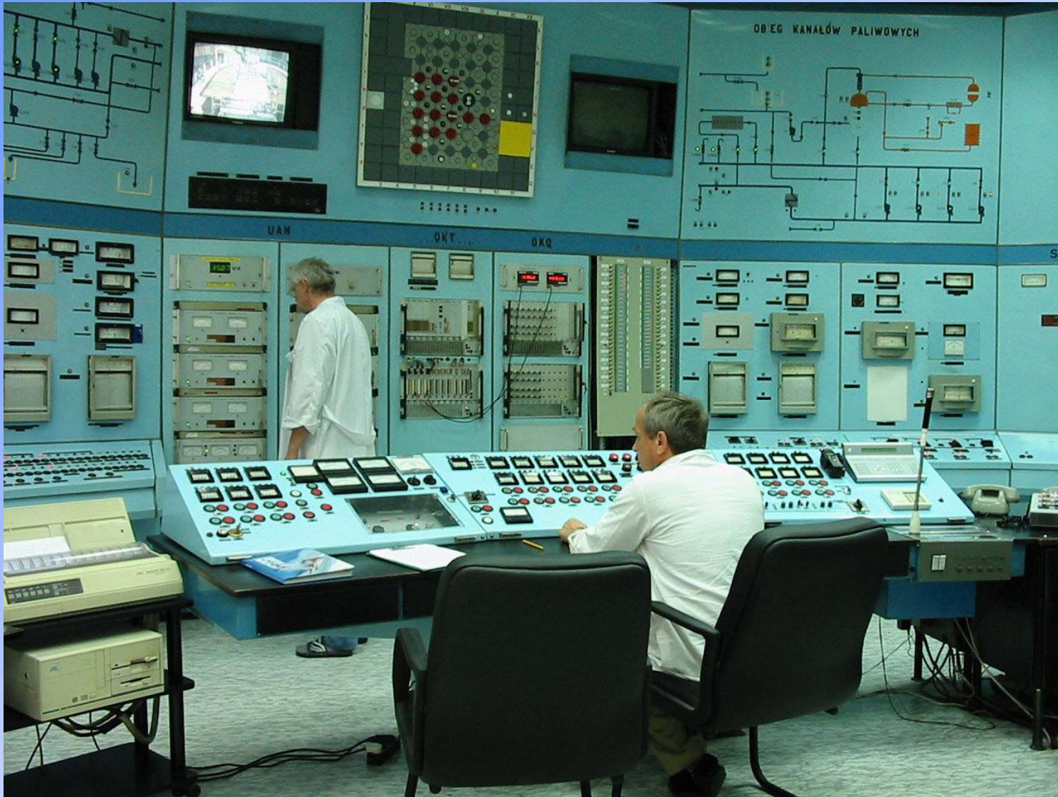
Control room of MARIA reactor
