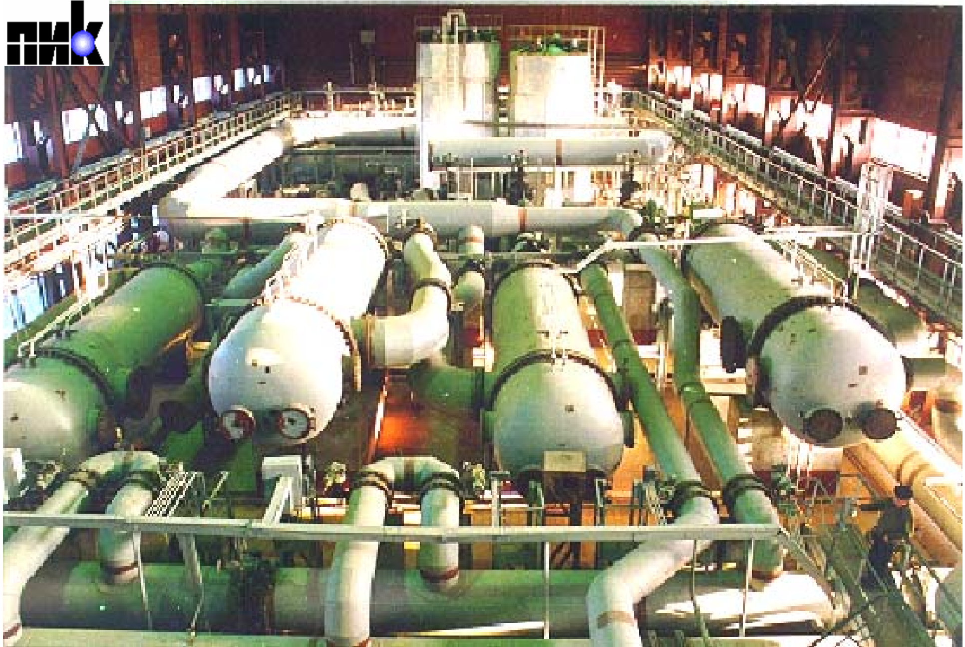
Secondary heat exchangers.
