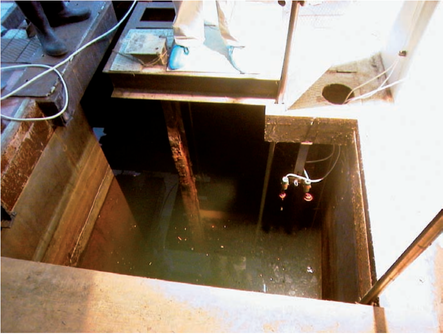
FIG. 7. Research reactor corrosion following an extended shutdown period.
