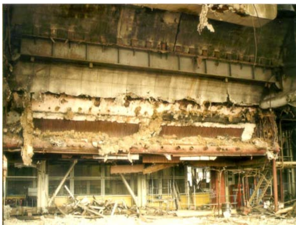
FIG. 5. The front of a large coal fired boiler from a power plant, partly dismantled without appropriate control.
