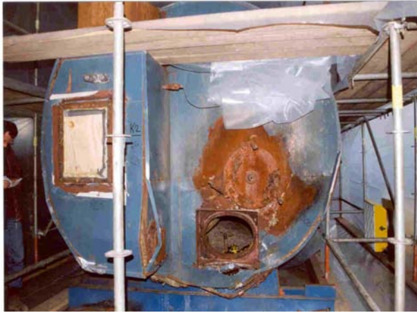
FIG. 3. A steam generator with slag wool under the corroded area.
