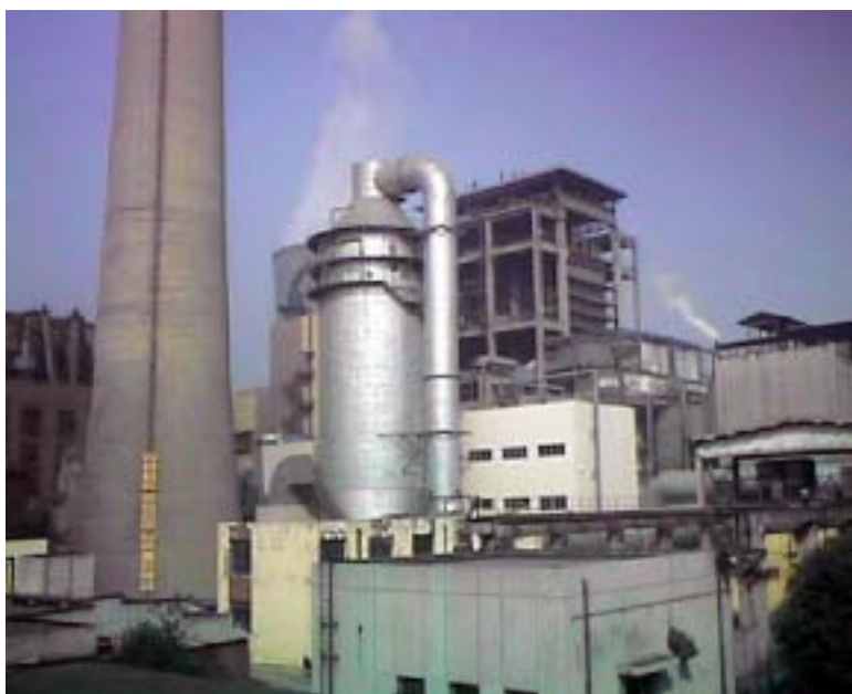
FIG. 6. A flue gas cleaning plant in Changdu, China.
