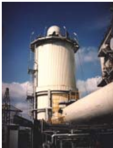
FIG. 3. Gas cooling tower.
