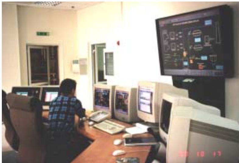
FIG. 1. Control room at EPS Pomorzany.
