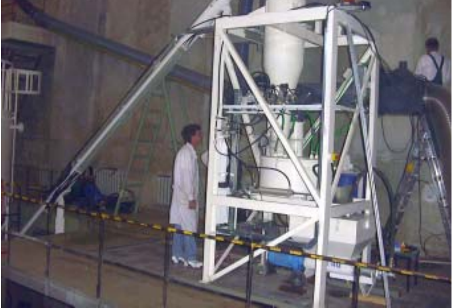
FIG. 11. Installation of the cementation plant in preparation for decommissioning of the Salaspils IRT reactor, Latvia.
