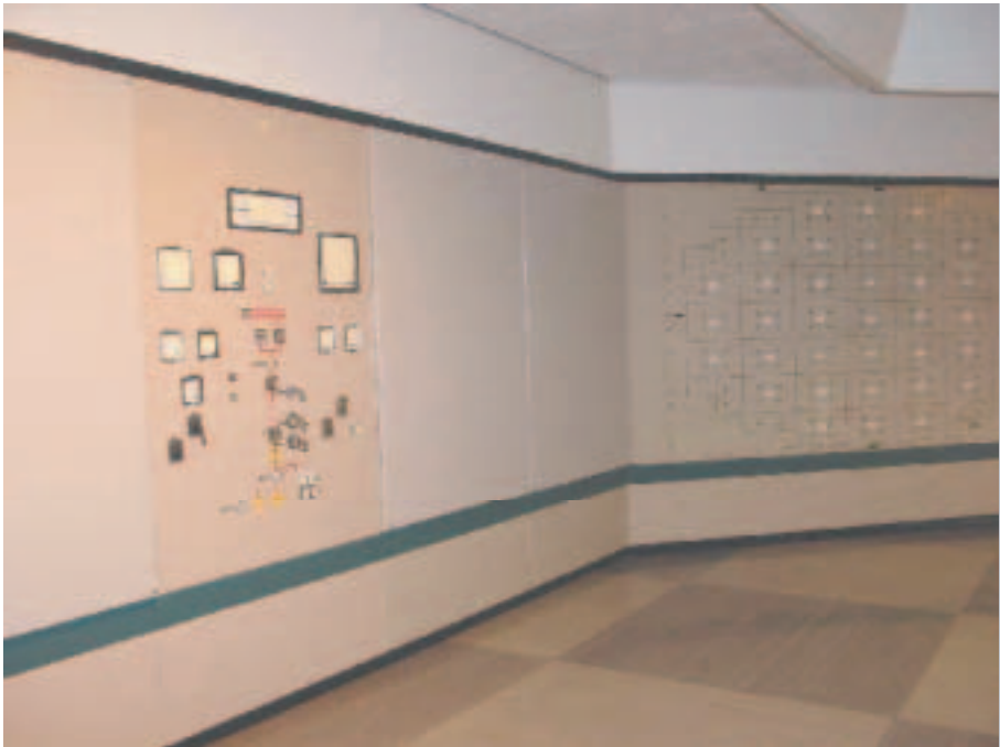
FIG. I-23. The control room of the Dodewaard NPP with inactive panels indicating that the systems are out of operation.
