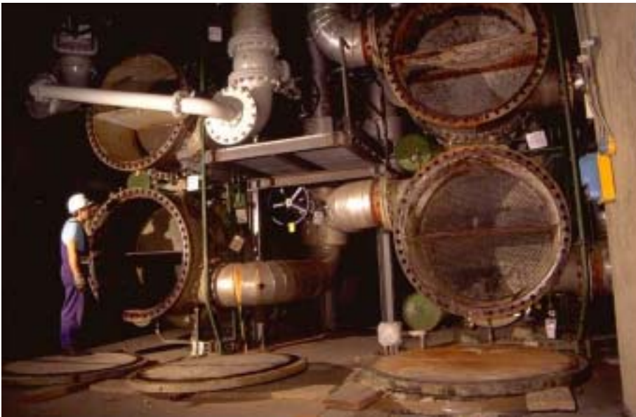
FIG. II-3. Caorso NPP heat exchanger.
