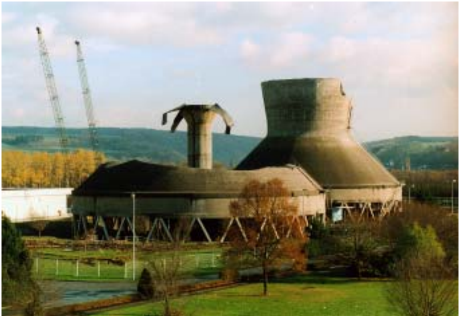
FIG. 13. Dismantling of cooling towers during the transition period at the Würgassen NPP, Germany.
