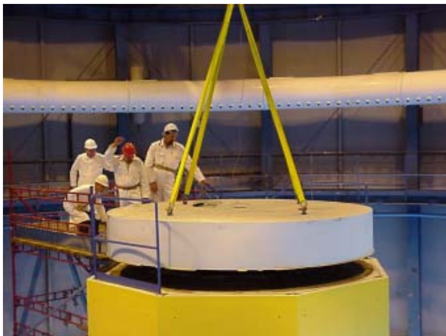
FIG. I-3. Twenty-five years after shutdown the concrete lid is lifted from the top of the DR-2 reactor, Denmark.
