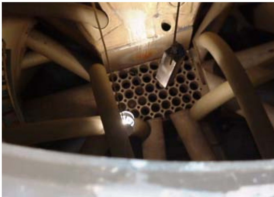
FIG. I-4. The last movable part, a beryllium reflector element, is lifted out of the reactor tank of the DR-2 reactor, Denmark.
