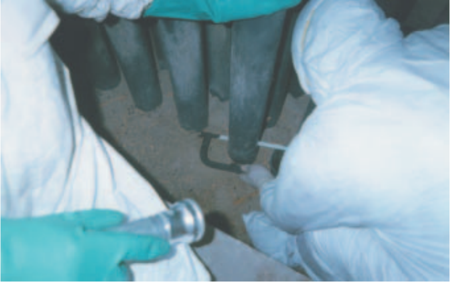
FIG. I.B-3. The pipes being cut at the lower level after the external surface contamination is measured. The contamination on the tools used was also checked.
