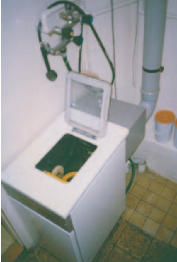
FIG. I.C-4. A device for emptying and washing urine pots.
