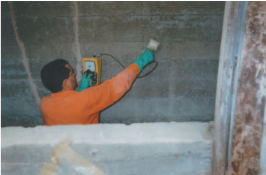
FIG. I.B-5. Final survey of the well after removing all radiation sources, pipes and sand. The measurements show the natural background levels.
