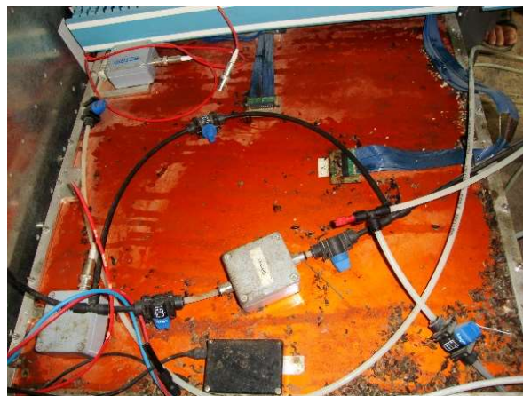
FIG. 36. View of a detector after 9 months of data acquisition in Khufu's Pyramid, showing degradation due to mice (courtesy of ScanPyramids 17 ).
