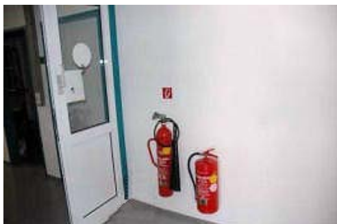
Fire extinguishers must be accessible and free from obstruction.
