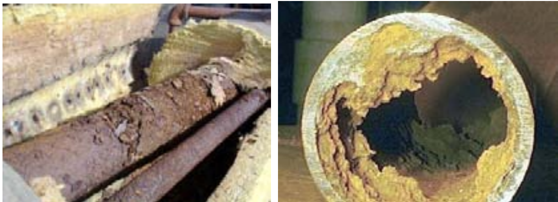
FIG. 16. Corrosion and deposit phenomena in piping system
