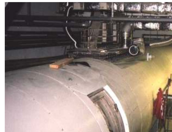
Industrial scale EBFGT Plant (~600,000Nm 3 /h)
