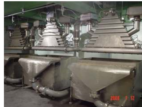
Industrial scale Wastewater Plant (10,000m 3 /day)
