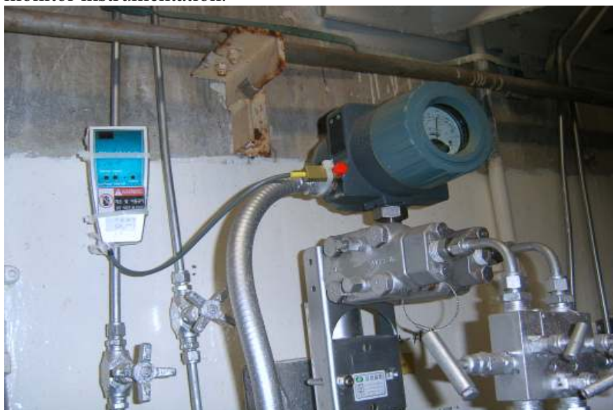
FIG. 1. On-line temperature monitoring system for cables and motors
