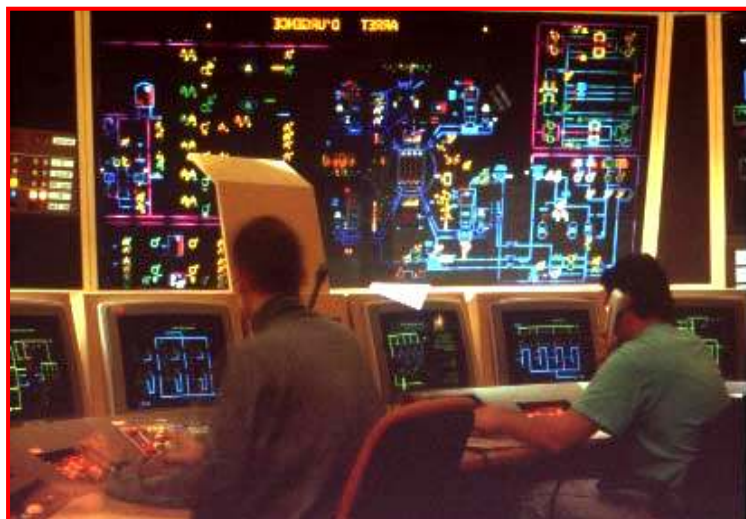
FIG. 9 Main Control Room (1500 MWe Unit)
