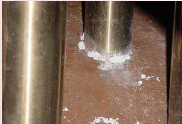
CRDM Penetrations Leaking
