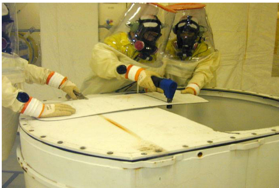
Workers wearing breathing air system and performing size reduction using a “nibbler” in the tent.
