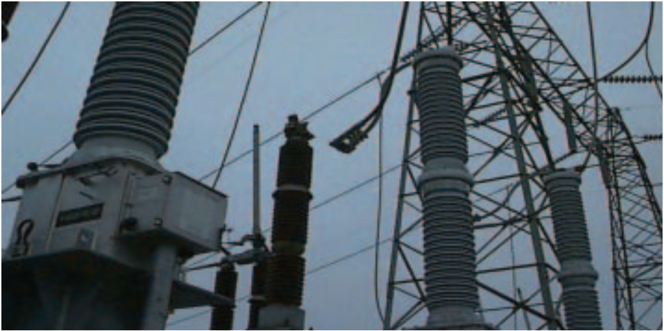
A 230 kV conductor on the jaw side of a disconnect switch was found broken and hanging freely (source: COG, Canada)
