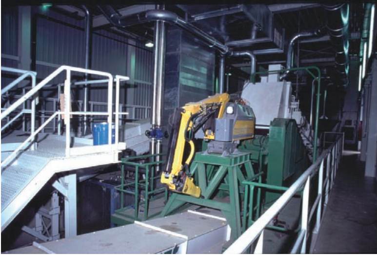
FIG. I-1.4. General view of the concrete crushing and sampling facility.
