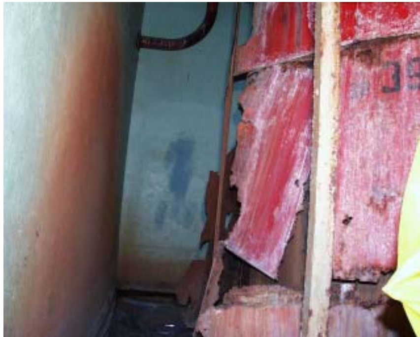
FIG. 15. A-1 NPP, Slovakia, waste treatment system; neutralization tank before decontamination and removal of the insulation.
