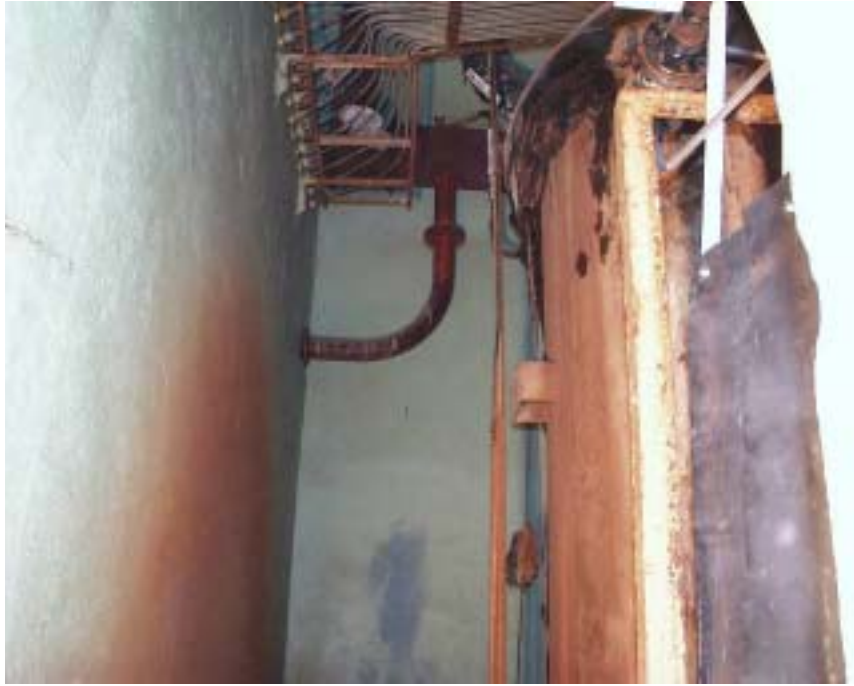
FIG. 16. A-1 NPP, Slovakia, waste treatment system; neutralization tank after decontamination and removal of the insulation.
