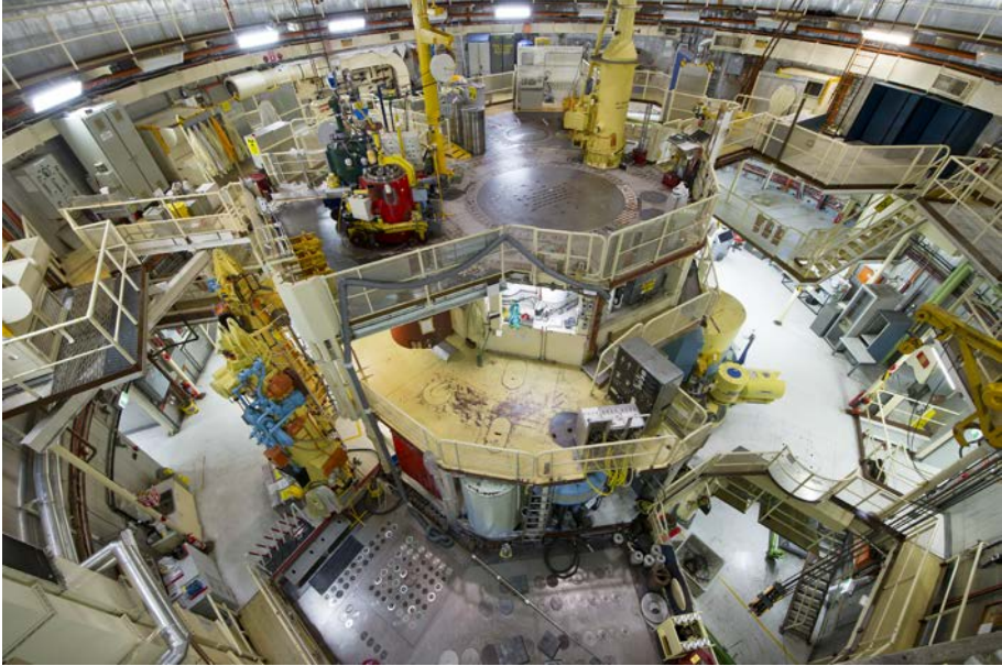
FIG. II-1. Internal image of the reactor containment building showing HIFAR and peripheral equipment (courtesy of A. Kimber, ANSTO, Australia).
