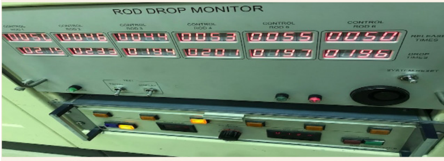
FIG. III-4. The old and new rod drop monitors installed to run in parallel for commissioning.
