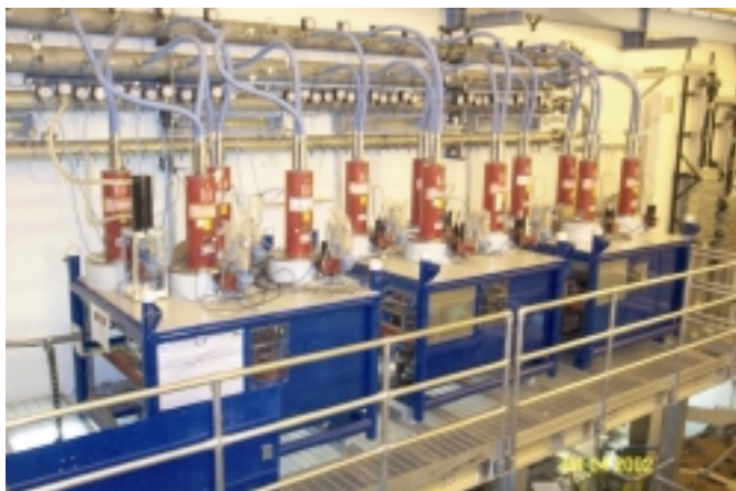
FIG. 16. Picture of 12 klystrons (4.6 GHz, 0.25 MW/unit) installed in the C-Mod experimental cell.
