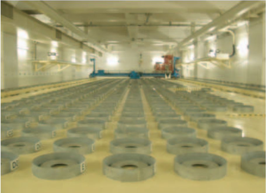
FIG. 4. JNC storage hall and the fully automated transfer system.
