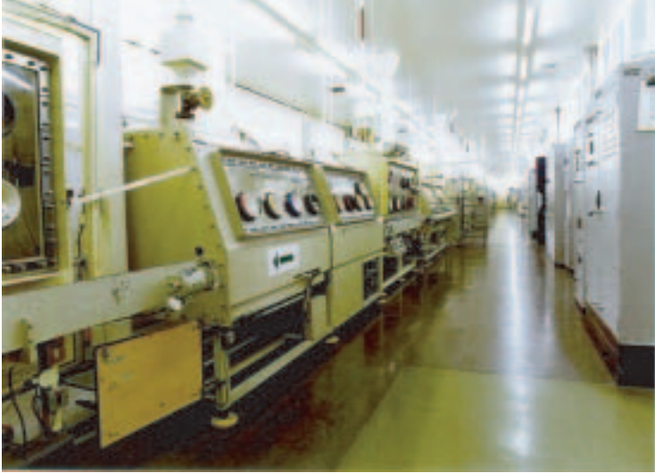
FIG. 25. The active canning line of the PFR fuel fabrication plant at Sellafield (before decommissioning).
