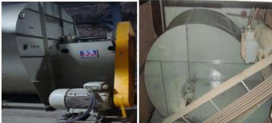
FIG. I-15. Replacement of aged rotating equipment like exhaust (courtesy of BARC, India)
