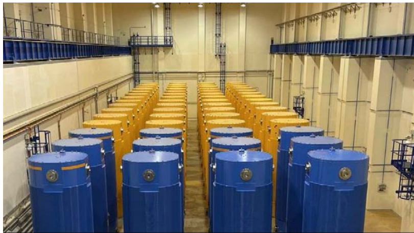
FIG.I-8. SF Dry storage containers (courtesy of SUJB, Czech Rep.)
