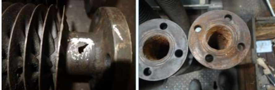
FIG. 13. (a) Hole in the heat exchanger (b) Rust in the heat exchanger (courtesy of NFC, India)
