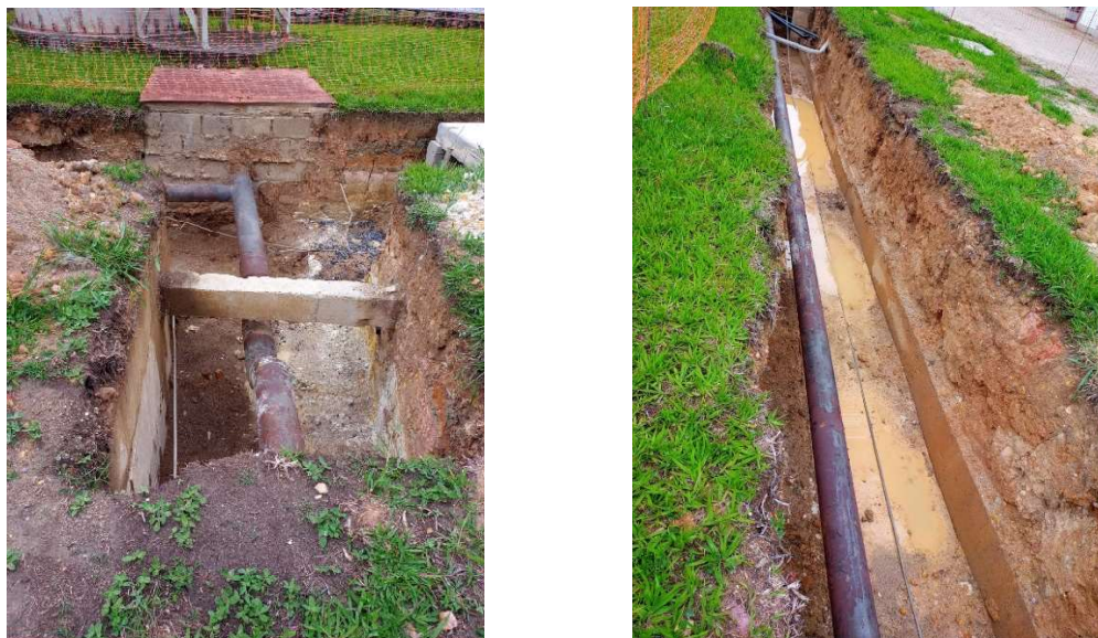
FIG. I-5. Old firefighting system (corroded condition)
