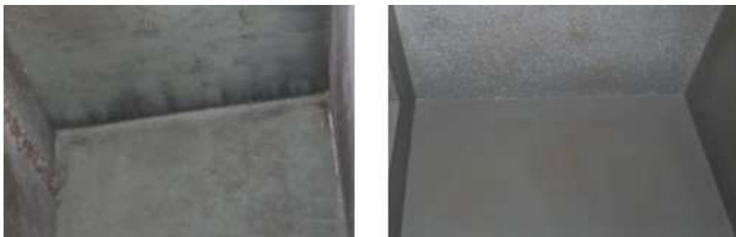
FIG. 9. (a) Crack in the concrete (b) Plugged crack (courtesy of NFC, India)
