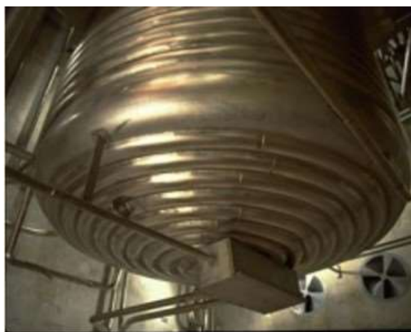
FIG. I-13. Evaporator at ORANO UP-800 facility (courtesy of ORANO)
