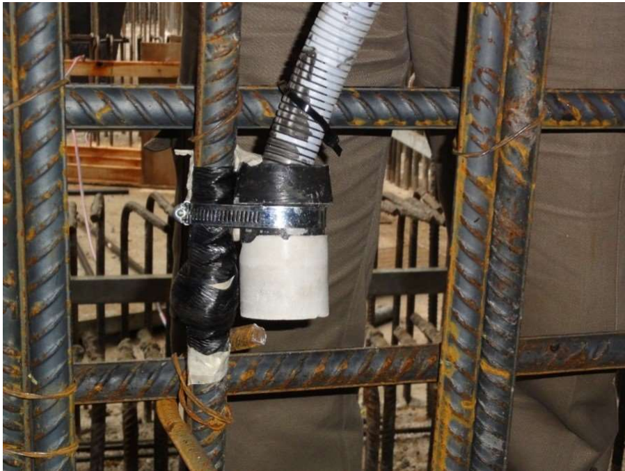
FIG. 6. Installation of probes for corrosion monitoring on steel reinforcement before concrete placement in the Dry Spent Fuel Storage Facility (courtesy of CNEA, Argentina)
