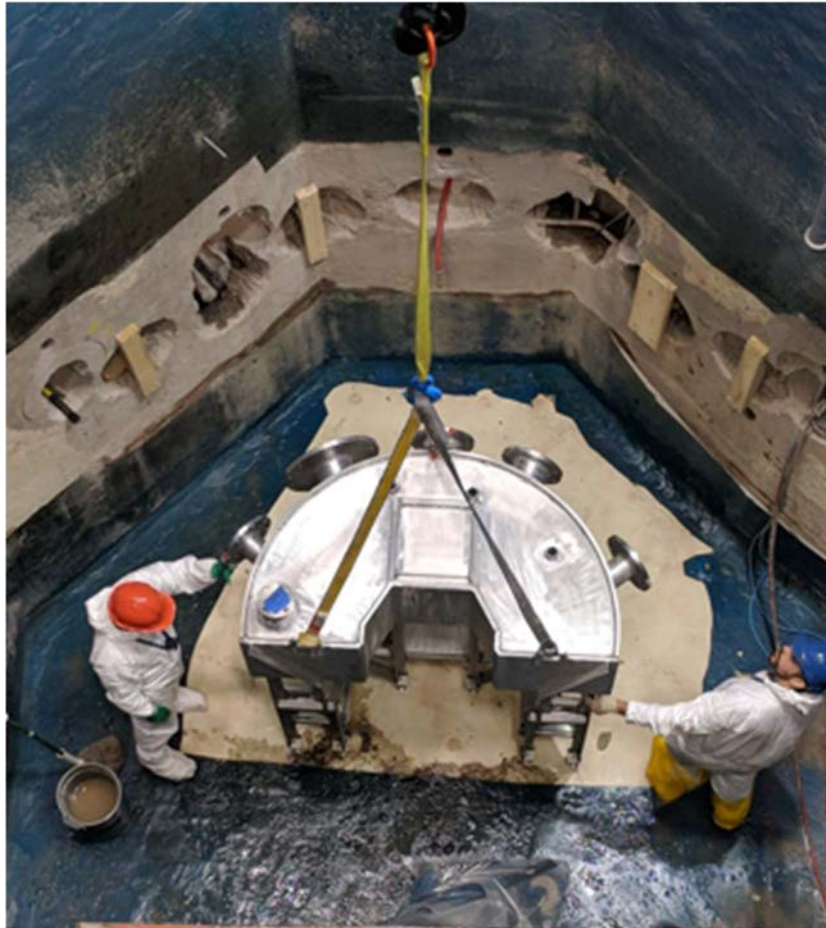
FIG. II-8. D_2O tank installation after taking out old beam ports and before installation of new beam ports (courtesy of K. Ünlü, PSBR).
