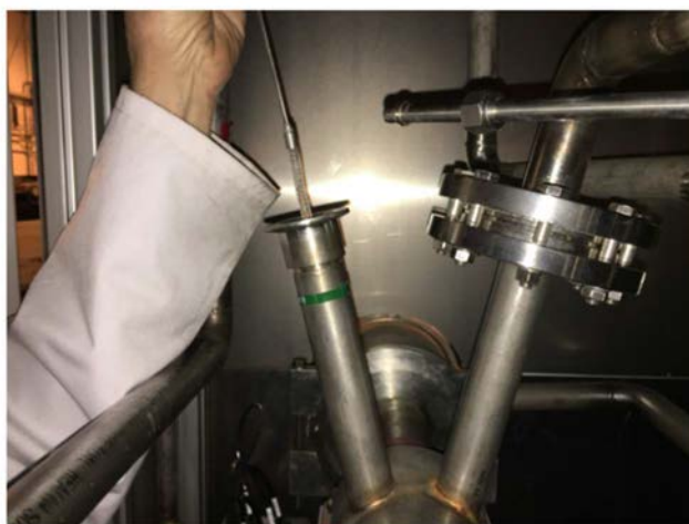
FIG. III-22. Ferric oxide catalyst mesh holder inspected in December 2015. This figure by the authors of Ref. [III-8] is licensed under CC BY-3.0.
