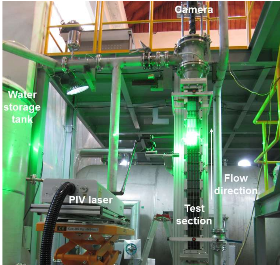
FIG. 4. Setup of the PIC system (Reproduced courtesy of KAERI [7]).
