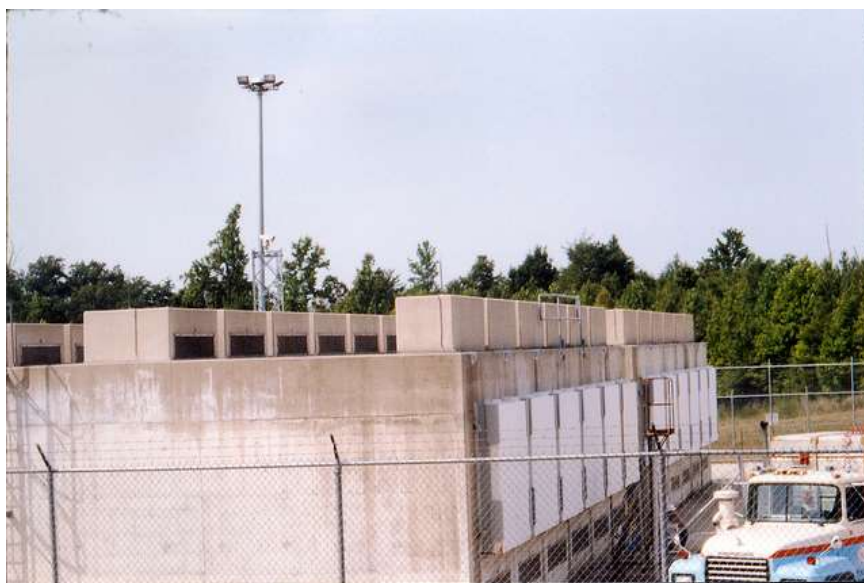
FIG. 8. NUHOMS ® system at Calvert Cliffs (photograph courtesy of US NRC File Photo).
