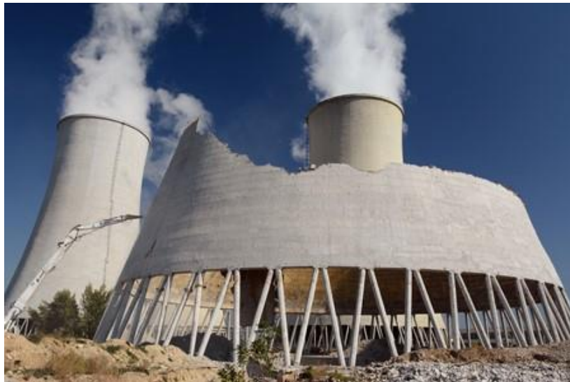
FIG. I-4. Demolition of the V1 NPP's four cooling towers. Note the operational cooling towers of the V2 NPP (photo courtesy of JAVYS, a.s.).
