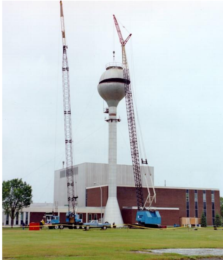
FIG. I-1. Dismantling of tank on top of the stack, WR-1 reactor, Canada (courtesy of WL).
