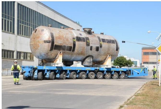
FIG. I-5. Transport of the steam generator for fragmentation in the turbine hall (photo courtesy of JAVYS, a.s.).
