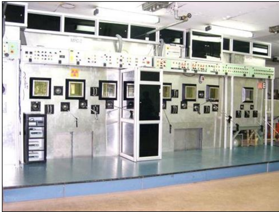
FIG. 2. Generator production facility.
