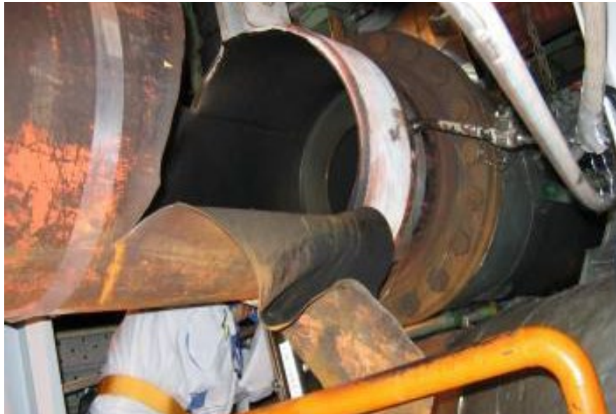
FIG. IV-23. Ruptured feedwater pipe (JNES, 2005).
