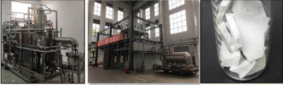
FIG. 9. Fluoride salts and production facilities (courtesy of Y. Zou, Shanghai Institute of Applied Physics).
