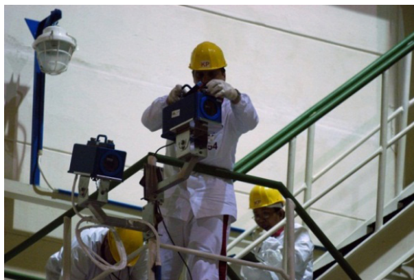
FIG. 10. Installation of a surveillance system.
