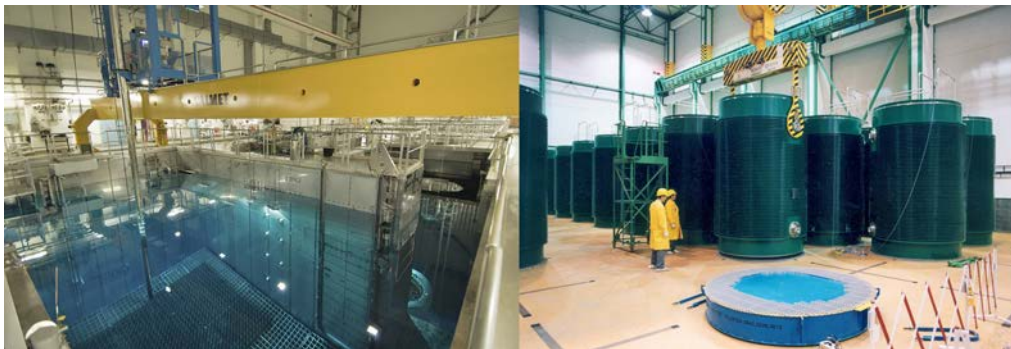
FIG. 8. Examples of wet and dry storage facilities: (left) Wet storage facility at the Olkiluoto nuclear power plant (Finland); (right) dry storage facility at the Dukovany nuclear power plant (Czech Republic).
