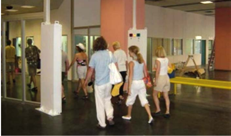
FIG. V-4. Example of a typical pedestrian RPM installed at a port.
