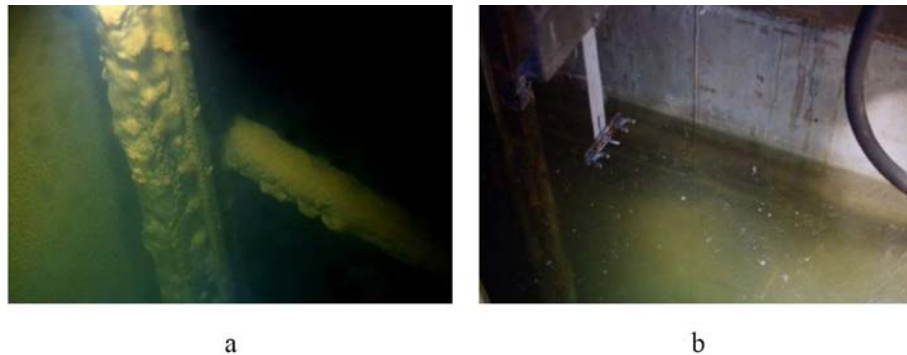
FIG. 32. (a) Corroded carbon steel structure inside of spent fuel storage pool and (b) floating dust on the surface of the AR pool [7].
