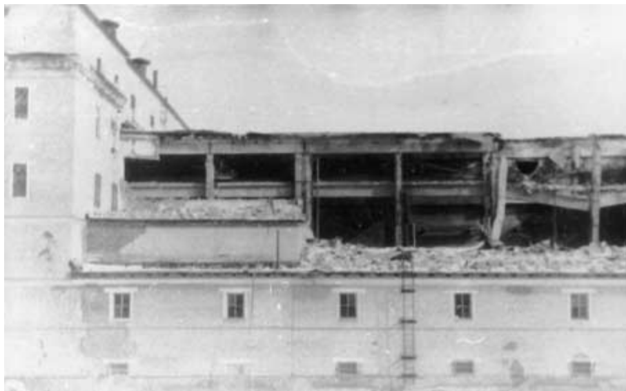
Photo 1. View of Building 201 after the accident.
