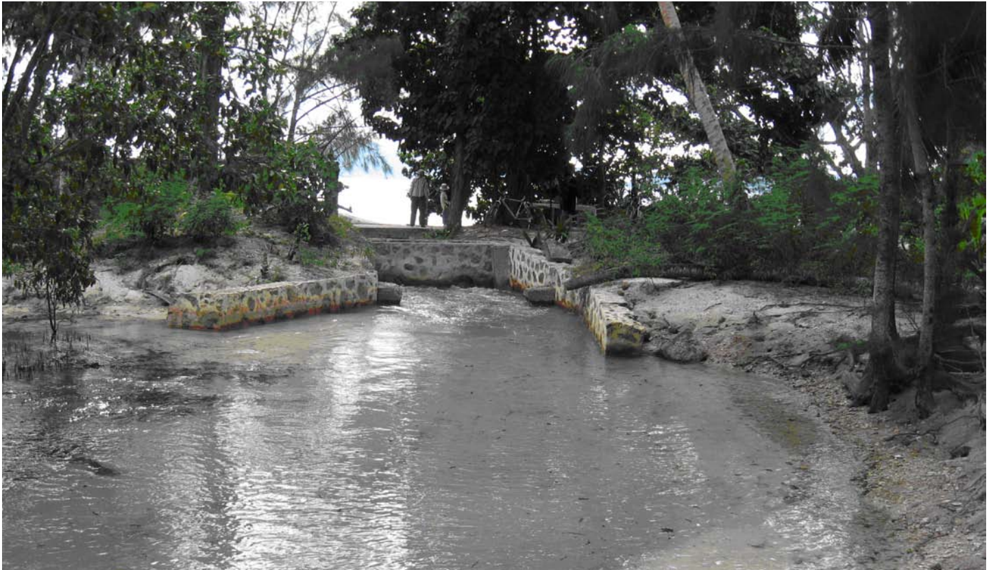
Sea water penetrating into the river channel during high tide. The river mouth was once equipped with non-return gates which prevented this ingress from occurring (Photo credit: E. Sacchi).
