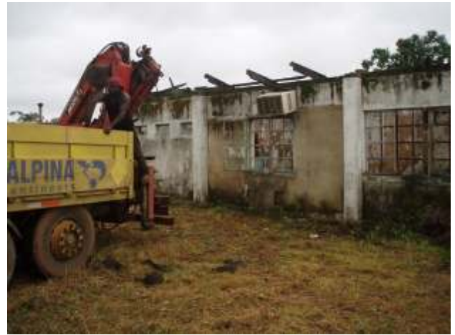
Crane in front of burned building housing sources at Vom
