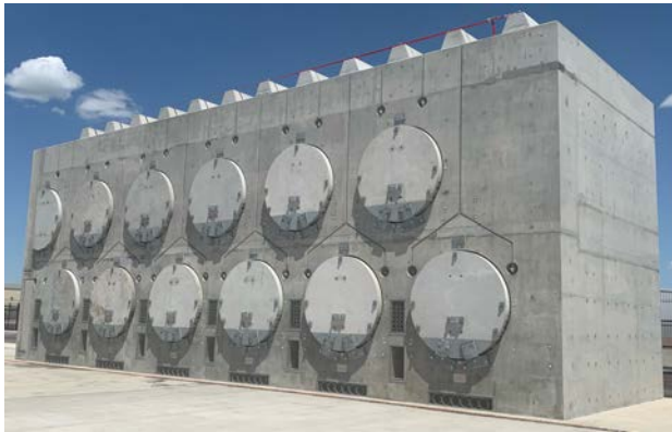
FIG. 36. Matrix system at Wolf Creek NPP (courtesy of Orano).
