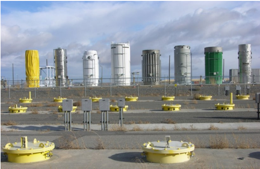
FIG. 15. Examples of different cask type at Idaho National Laboratory, USA.
