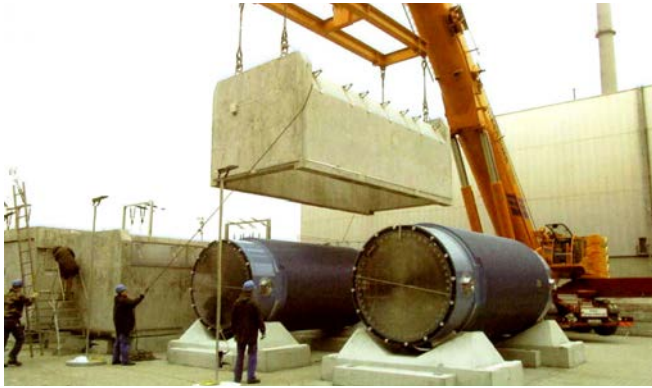
FIG. 20. Temporary horizontal storage in Germany (courtesy of Gesellschaft für Nuklear-Service).
