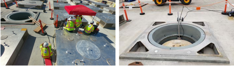
FIG. 70. Inspections of UMAX MPC system at SONGS: inspection crew set-up (left) and robot with high-resolution camera deployed inside of the UMAX storage module (right). (Courtesy of SCE.)
