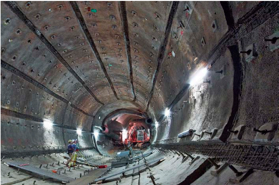
FIG. 25. Waste transportation tunnel under construction at the Konrad Repository in Salzgitter, Germany. Reproduced courtesy of the Bundesgesellschaft für Endlagerung mbH.
