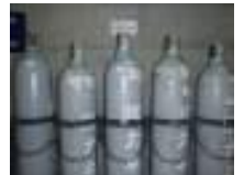
Back-up Battery and Cylinder
