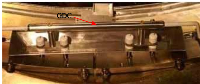
FIG.4. GDC Installed in EAST VV.
