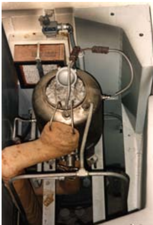
Fig. 3 The recombiner seen from above.
