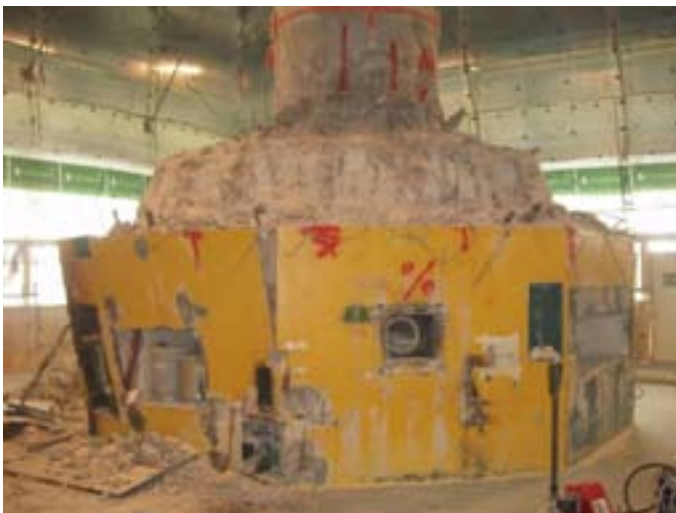
Fig. 23 Lower part, steel face plates being removed. Horizontal tubes cut out with wire.
