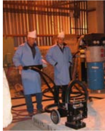
Fig. 16. PENTEC VAC-PAC System with Squirrel II decontamination tool.
