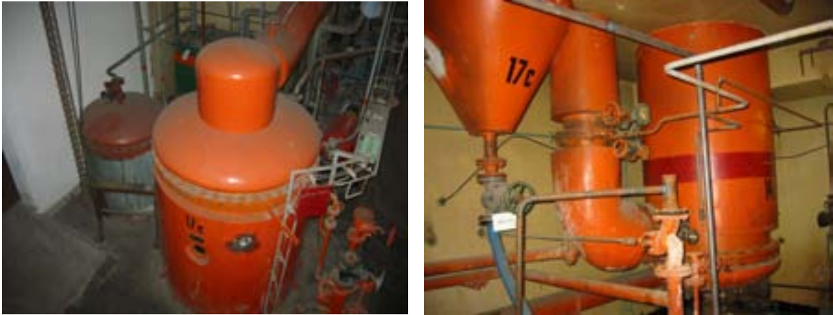
Fig. 9. Old evaporator (upper and lower parts).
