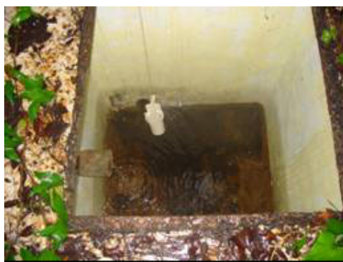
Fig. 8. Retention tank for collection of liquid effluents at the WPF.
