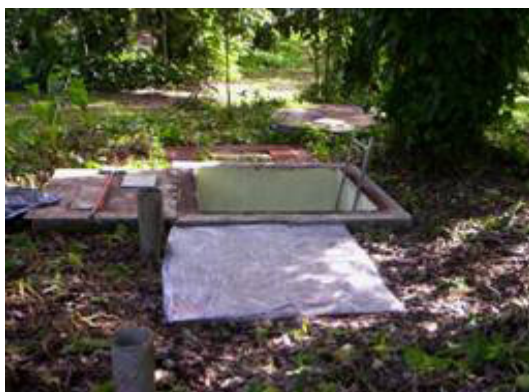
Fig. 12. Control area prepared for characterization and D&D operations in the retention tank.
