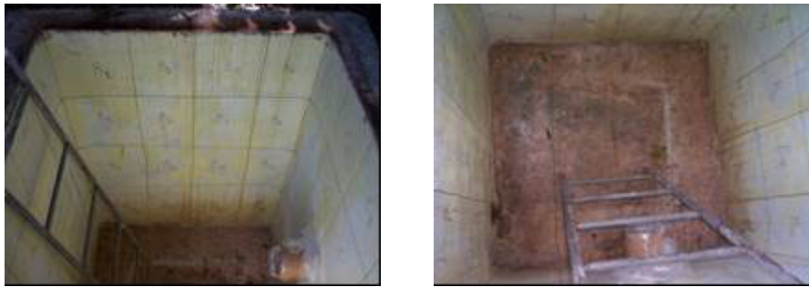
Fig. 14. Preparing the walls and floor of the retention tank for radiological survey.
