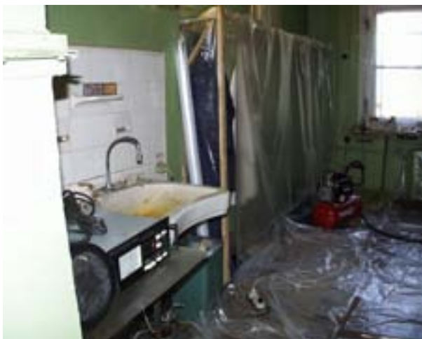
Fig. 11. Example of temporary sanitary dosimetric post in the room.
