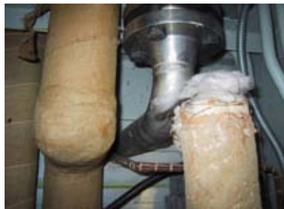
Fig. 4 Flange at the bottom of the recombiner.
