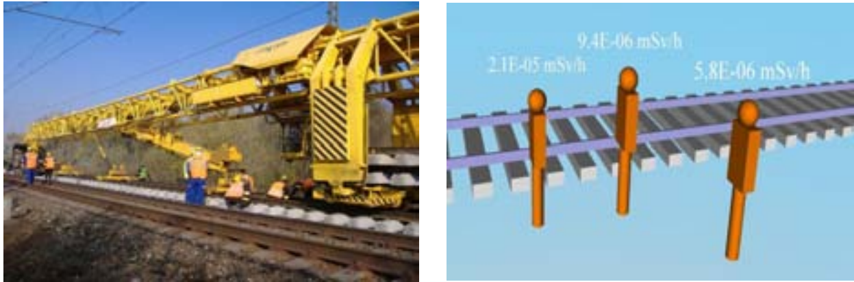
Fig. 19. Example of modelling - installing the rails on site and the model in Visiplan software.
