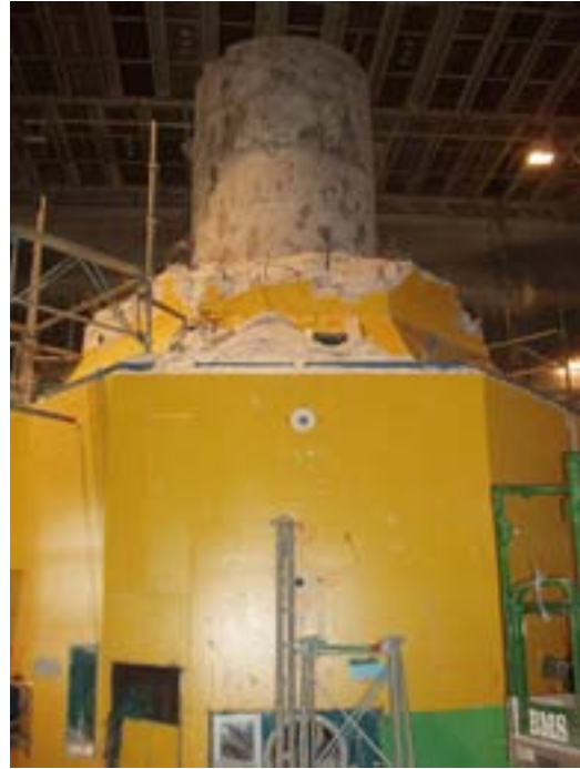
Fig. 22 Chimney down, reactor tank exposed.
