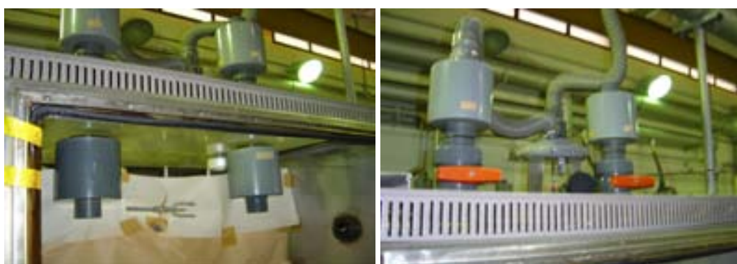
Fig.16. HEPA filters for assembling in the glove-box.
