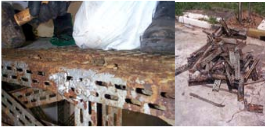
Fig.20. Corroded perforated carbon steel structures before and after dismantling.
